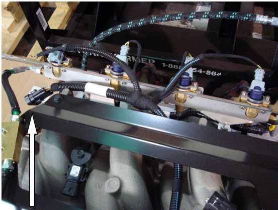
This is how the injector harness connector is currently oriented. Photo also shows driver's side harness routed over the stamped steel injector rail,
