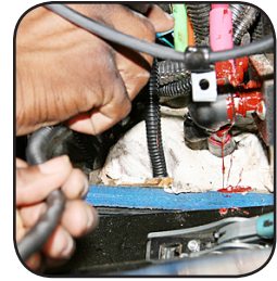
Wiring Access to Chassis
