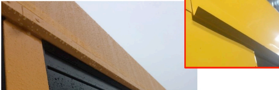
Figure 3: The esthetical aspect of the former drip rail installation, with bottom sealed with the windows top
